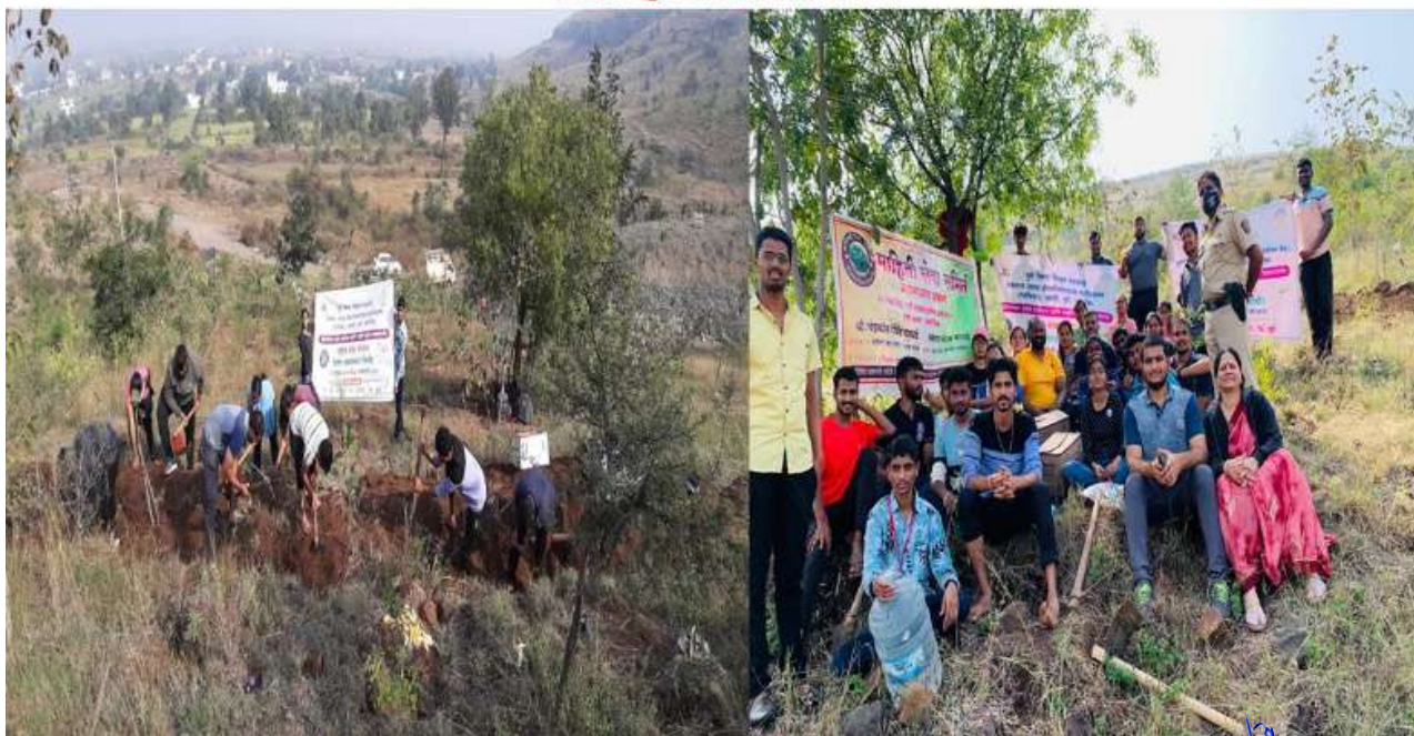
Work for the purpose of water conservation and water horizontally by digging continuous counter trenches(CCT) on the Bakori hills.
